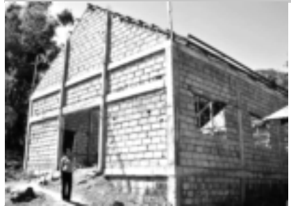
Anabaptist Mennonite Community Church, Pantabangan, Nueva Ecija, pastored by Bishop Adriano Fernandez. Yda Villa, former youth leader, stands in front of the church building that is currently being expanded.
